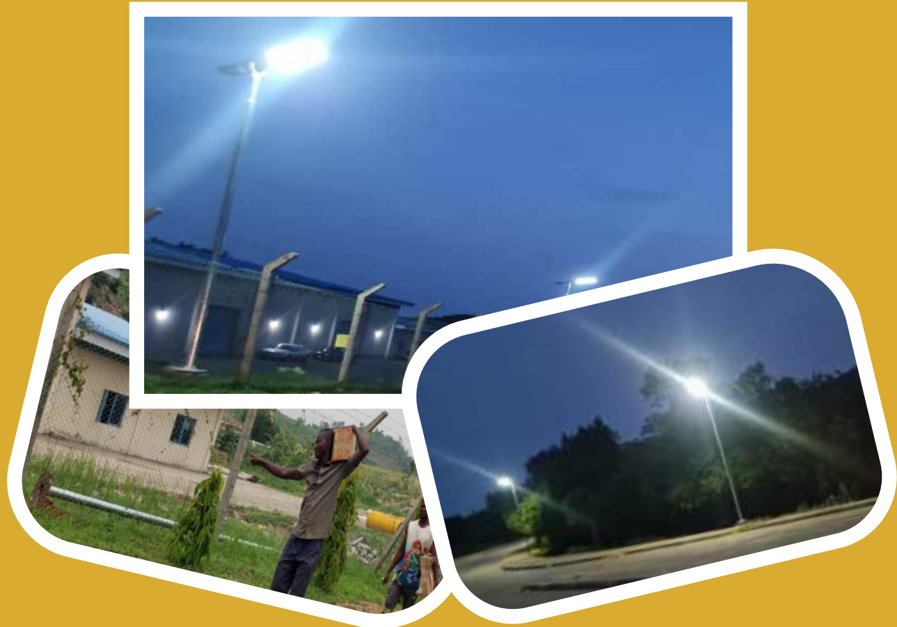
INSTALLATION OF SOLAR STREET LIGHT PROJECT AT LOWER USMAN DAM MAIN JUNCTION
