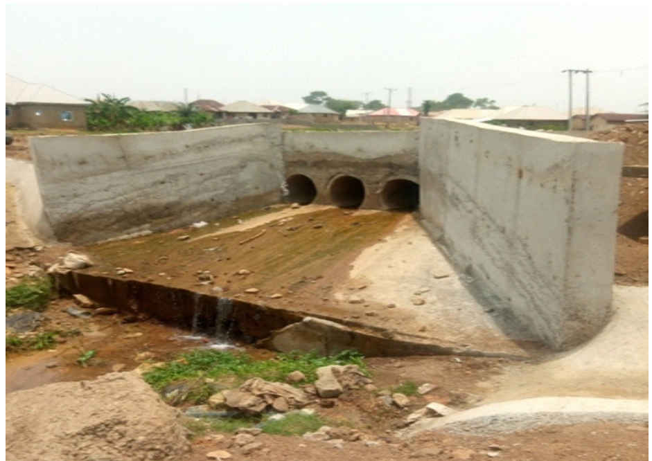
RECONSTRUCTION OF BOX CULVERT ACROSS STREAM AND PIPE CORRIDORS PROJECT IN DUTSE SOKALE AND JIWA
